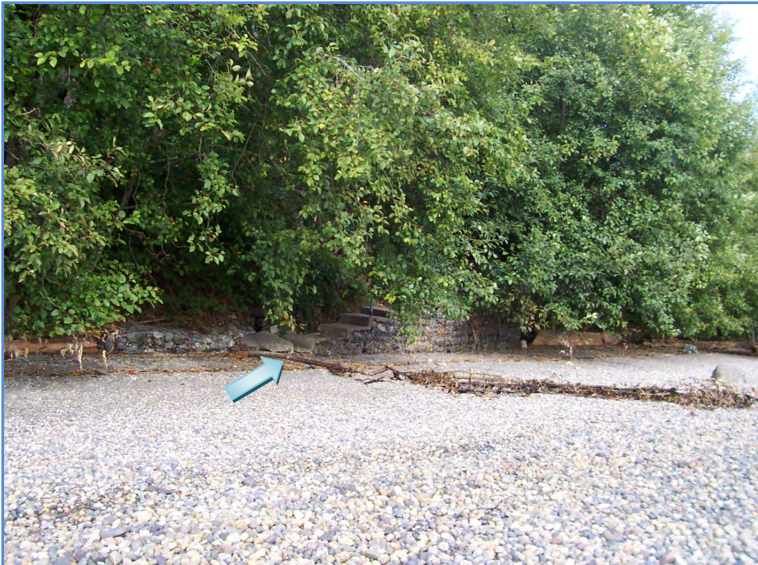
Figure 7.6. Ground photo (SPSSEG 2009) of concrete and gabion bulkhead at Maple Hollow Park.
